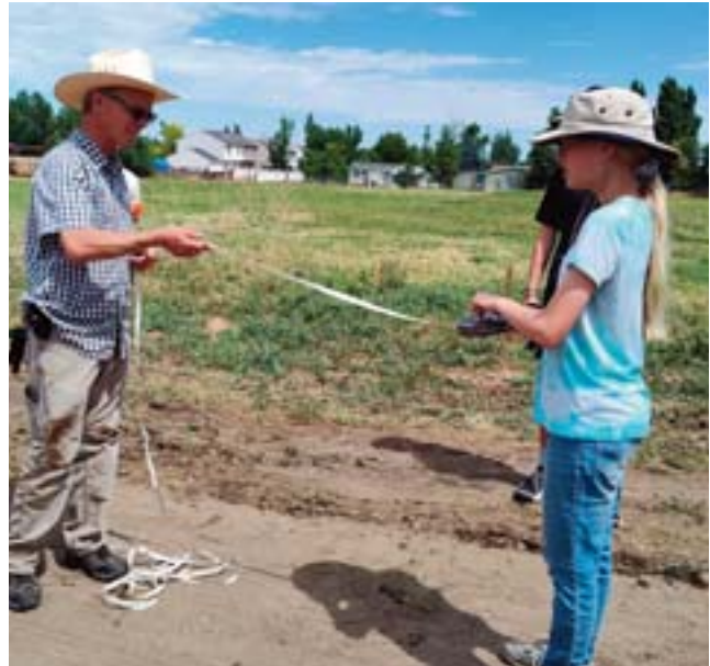
Nicole Loewen (right) and her father, Jonathan Loewen, measure the distance for new fence post holes to be dug during a work project for a couple at Lakeview Church. Photo by: Jody Burkett.
